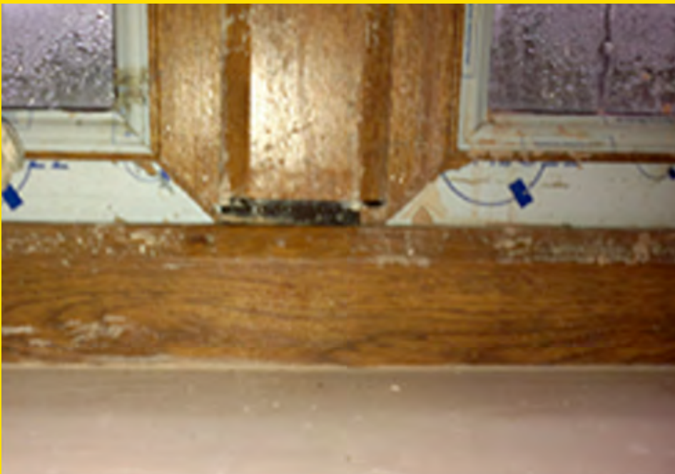
Surface condensation on windows due to heat loss through the windows and the incorrect levels of ventilation
