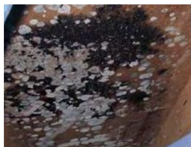
Showing interstitial condensation resulting with mould through the wall.
